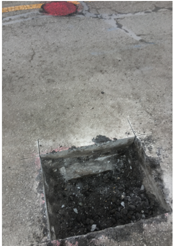
A cut made on West 96th Street by Jim Swift, PS, of the Boone County Surveyor’s Office advanced a search by Norman Hiselman, PS, of Weihe Engineers, Inc., for a stone that marked the quarter corner on a line in Township 17 North, Range 2 East between Section 14 in Marion County and Section 11 in Boone County. The stone was found at a point 7.46 feet south of the previously referenced Harrison marker, which is spray-painted pink at the top of the image. (Photo provided by Jim Swift)
