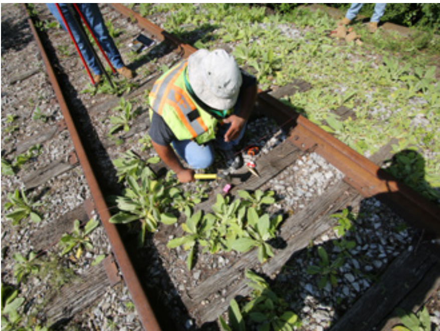
Crew chief Robert Pangelinan sets a MAG nail at the intersection of the centerline of a culvert and the centerline of the former Nickel Plate Railroad tracks. Marion County Surveyor's Office crews recorded 152 locations between 96th and 22nd streets. Photographer Ethan Evans' shadow is at right.
