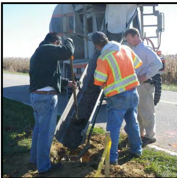
L. to R.: Calvin Cash, Matt Badger and Greg Kissel pour concrete into a form for one of the marks. Photos provided by Matt Badger.
