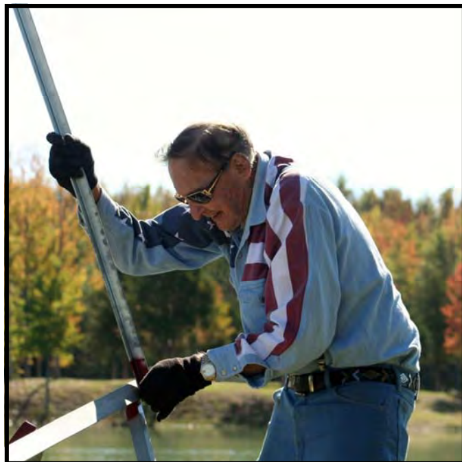
Ulis Jones, the hardest-working man on the ground, and sometimes on the tower, during the erecting of the Bilby Tower in Osgood Park, Osgood, Indiana.
