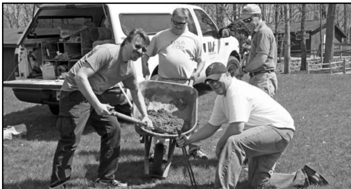
Preparing to put concrete into one of the five 36-inch-deep holes dug April 18 to mark corner positions at the new Surveying Merit Badge course at Belzer Scout Camp are (clockwise, from left) ISPLS volunteers Maciej Zurawski; Mark Schepers, PLS; David York, PLS; and Ryan Swingley, PLS. The two pieces of rebar in Swingley’s hand will allow the monument to be found by a metal detector. The installation phase took about 2-1/2 hours.
