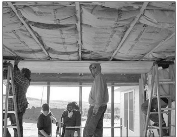
Installing ceiling insulation in the reconstructed home of Dolores Stevens in Greensburg, Kansas are Friends Disaster Service team members (left to right) Donald W. Wimmer; L.S. ISPLS member, Amada Ridge, Lisa Wimmer, ISPLS Associate member, and Dolores Stevens' grandson Brennan and Jimmy. Image is courtesy of Lisa Wimmer.
