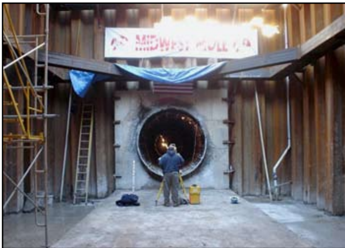
Sean Murphy of USI Consultants, Inc. is checking the centerline stationing and the as-built information from the south to the north of the 2014-foot long Indianapolis International Airport utility corridor tunnel. Image is courtesy of USI Consultants, Inc.
