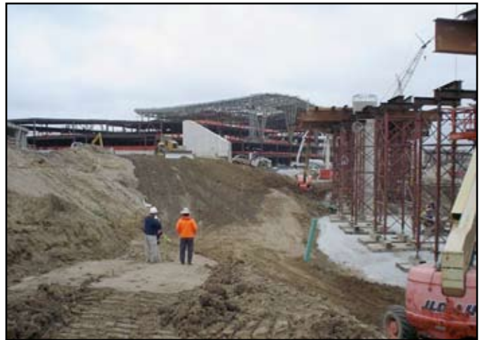
George Starks (left) of USI Consultants, Inc. and project contractor confer on the Indianapolis International Airport expansion mass grading construction staking. Image is courtesy of USI Consultants, Inc.
