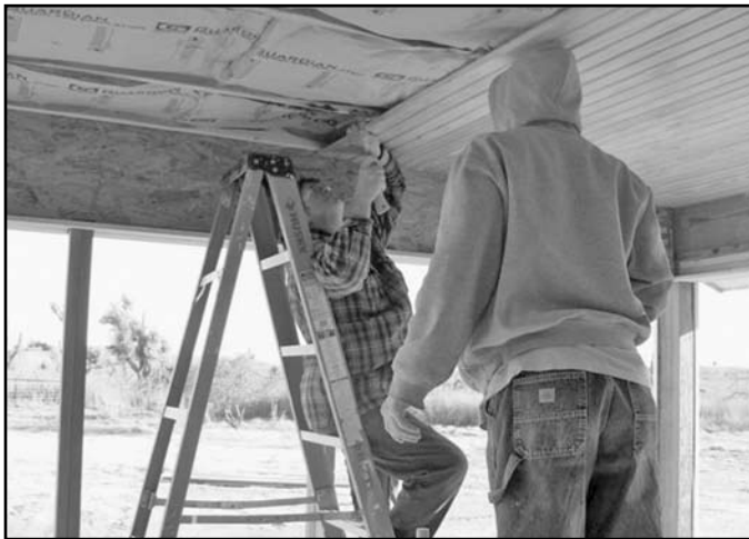
Donald W. Wimmer, P.L.S. ISPLS member (left) and Dolores Stevens' grandson Brennan install the devetailed wood ceiling in the porch of the reconstructed Stevens' home destroyed by a May 5, 2007 tornado in Greensburg, Kansas.
