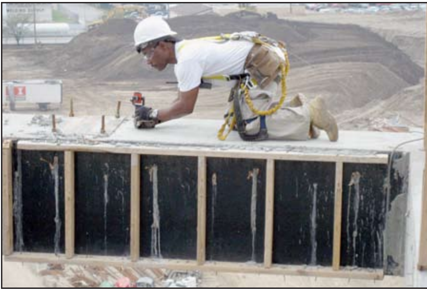
Meddie Demmings of Benchmark Land Services, wearing a protective harness attached to a safety cable, is setting out a column line in preparation for measuring as-builts of the anchor bolts at the southeast corner of the Lucas Oil Stadium. Note about 140 feet below the concrete beam the size in apparent miniature of materials and equipment on the playing field level of the stadium.
