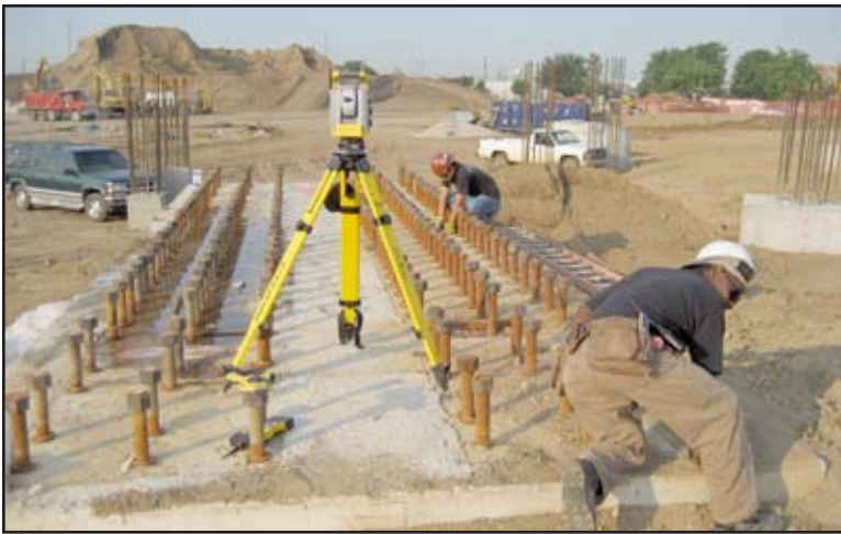
Meddie Demmings of Benchmark Land Services (foreground) is assisted by Daniel Pearson of Derr Steel Erection Company of Euless, Texas in conducting the as-built measurement of the shear wall anchor bolts at the southeast corner of the Lucas Oil Stadium. There are 180 anchor bolts in this configuration. Precise locations of the anchor bolts are required for the fabrication of a steel plate to be placed over the anchor bolts.
