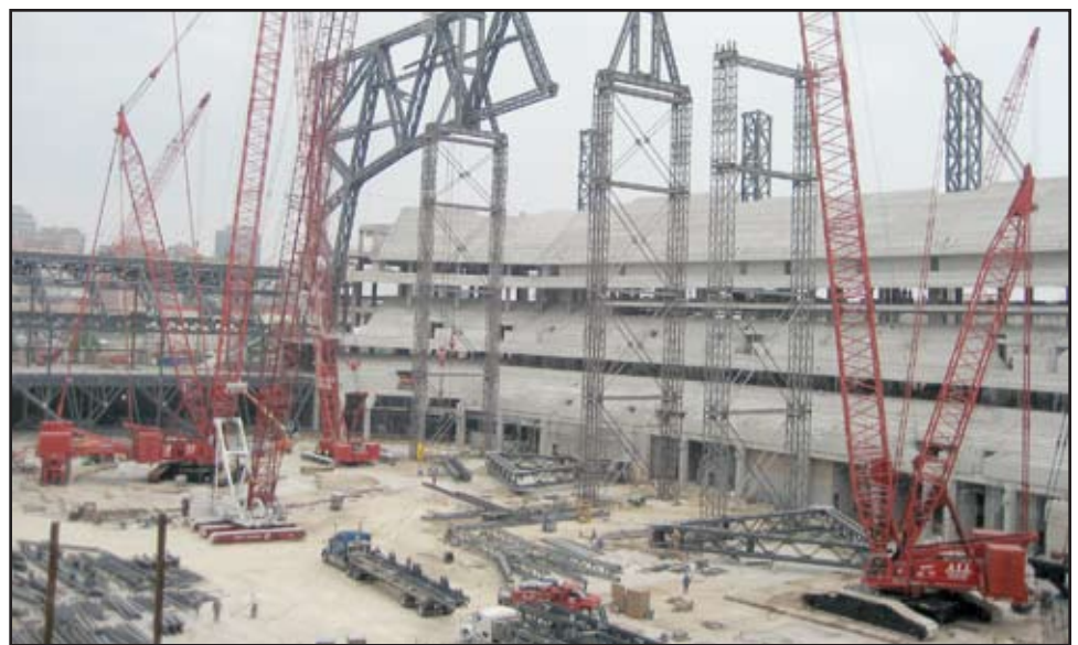
Above is a view of the northeast corner of the Lucas Oil Stadium under construction in Indianapolis highlighted by the initial placement of the north end of the east super truss. When completed the two super trusses that will support the moveable roof will measure 752 feet in length each with clear spans of 629 feet.
