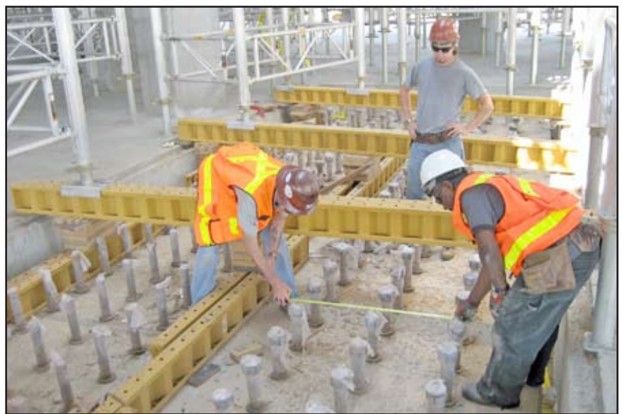
William "Buckshort" Shackleford of Derr Steel Erection Company (left) and Meddie Demmings of Benchmark Land Services run check measurements of anchor bolts with Daniel Pearson, also of Derr, observing, before commencing with the anchor bolt final as-built measurements on the shear wall at the southeast corner of the Lucas Oil Stadium, Note the temporary beams supporting temporary scaffolding.
